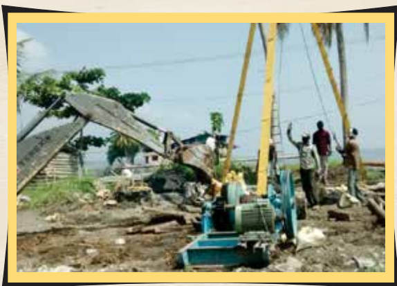
Pile Foundation Works for Boys, Girls Hostels and Dining Hall at Sai, SAG Centre, Alleppey Kerala.
