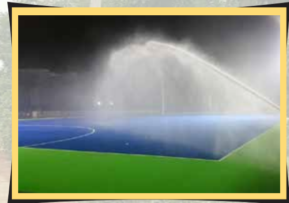
Relaying of Global Category Synthetic Hockey Surface-II(Blue Turf) & Automatic Sprinkler System At Sai, Bengaluru.
